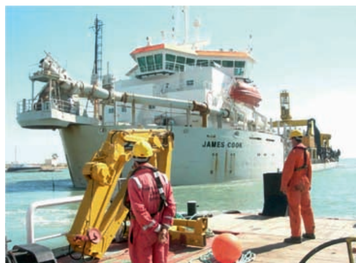
Figure 7. Connecting floating pipelines to the TSHD James Cook for the rehabilitation works.
